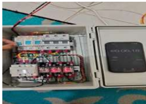
Figure 1. R Phase ON to OFF Test
