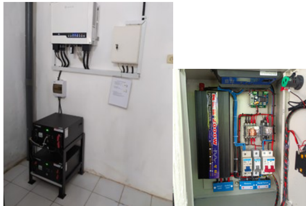
Figure 6. Battery and PV Junction Box
