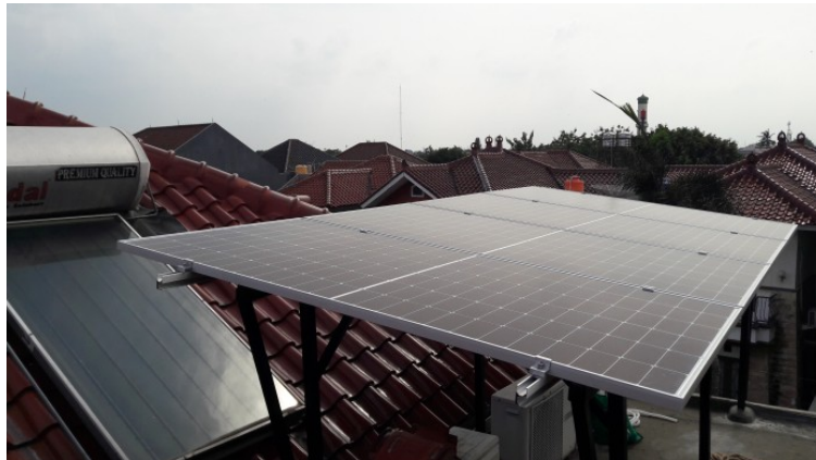
Figure 5. Solar Panels Installed
