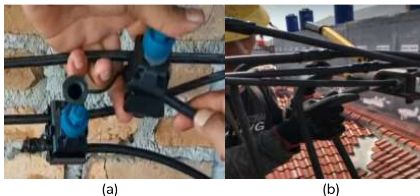
Figure 4. (a) Connection Point Using Connector Tap. (b) Connection Point Using Joint Press Connector
